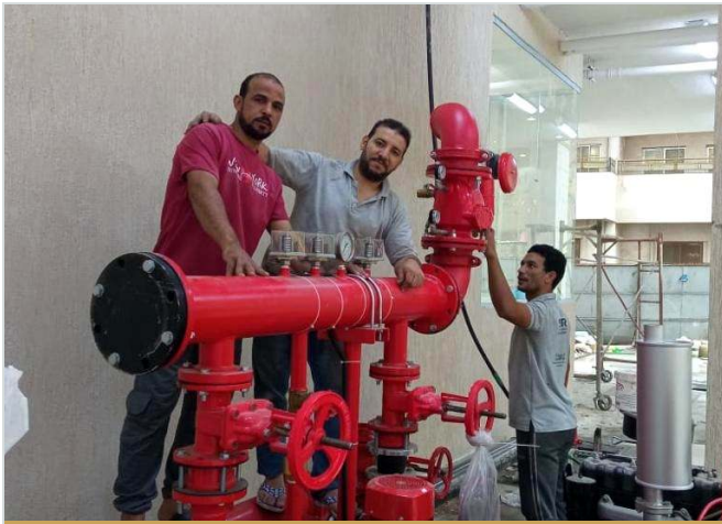
Fire-Pump Room Installation NDC Site — Firefighting Pump Skids & Piping
