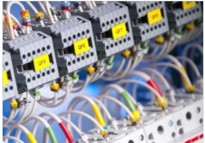
Electrical Distribution Panels Power Distribution & Control Works
