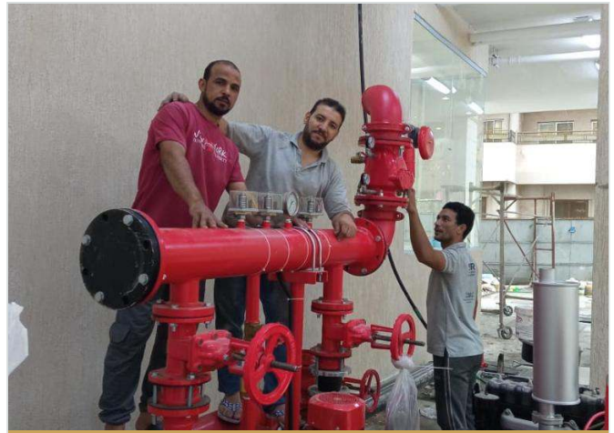
Pump Room Commissioning Team NDC Engineers & Technicians On Site
